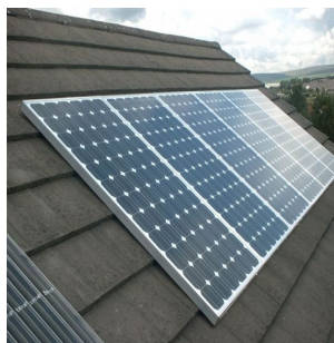
Solar PV Panel
